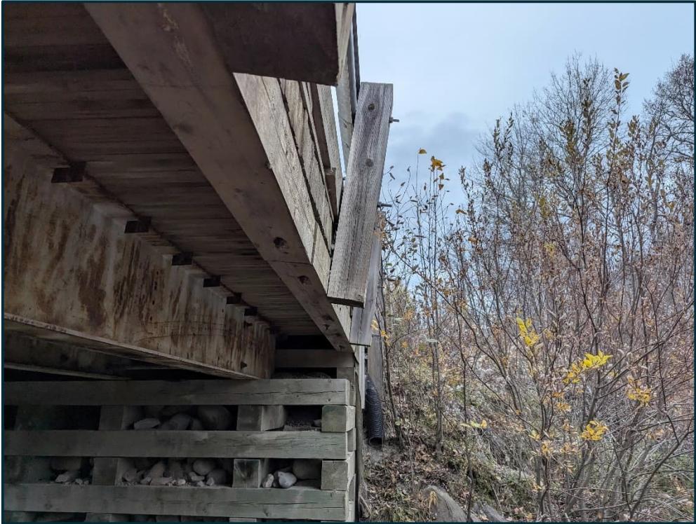
8. B-030 2024-10-23 Barrier Post Leaning
