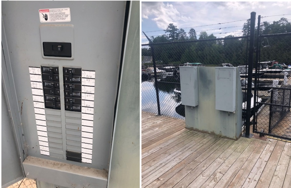
Figure 1 – Existing 200 A Electrical Panel
