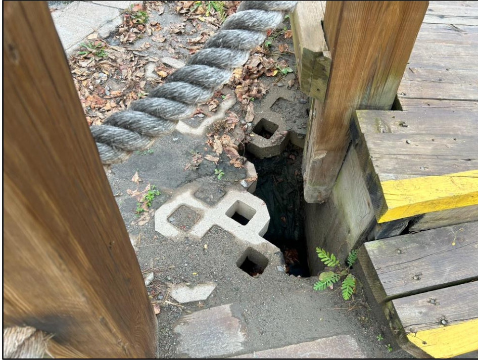
Photo 25: General soil movement at drainage pavers near east end stair adjacent of gas pump.
