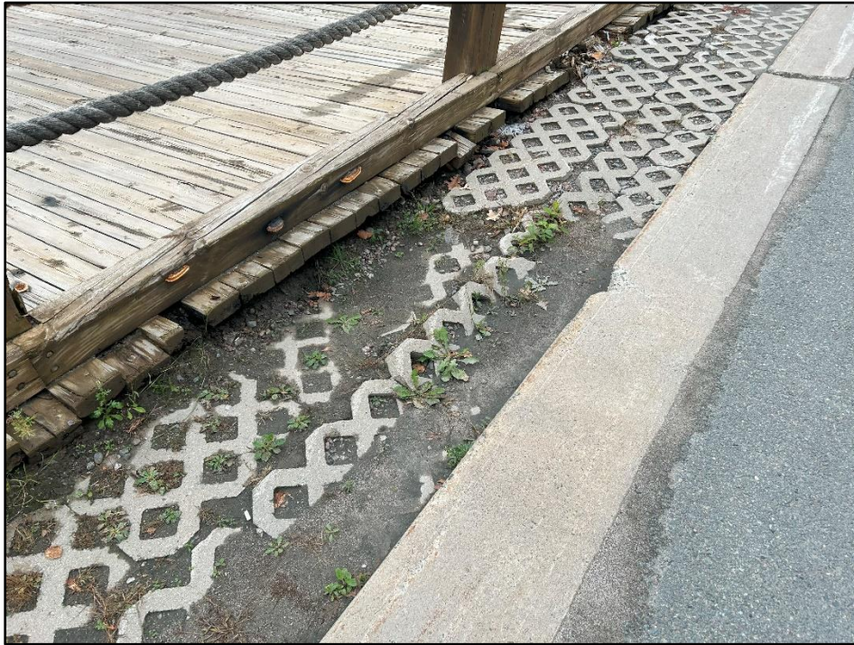
Photo 23: General soil movement at drainage pavers.
