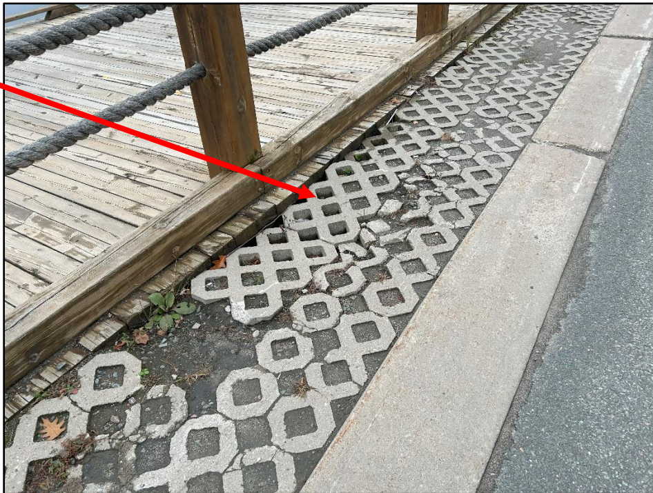
Photo 24: General soil movement at drainage pavers.
