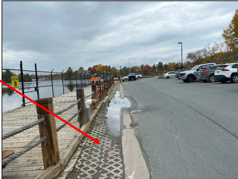
Photo 21: Pooling water on drainage pavers.
