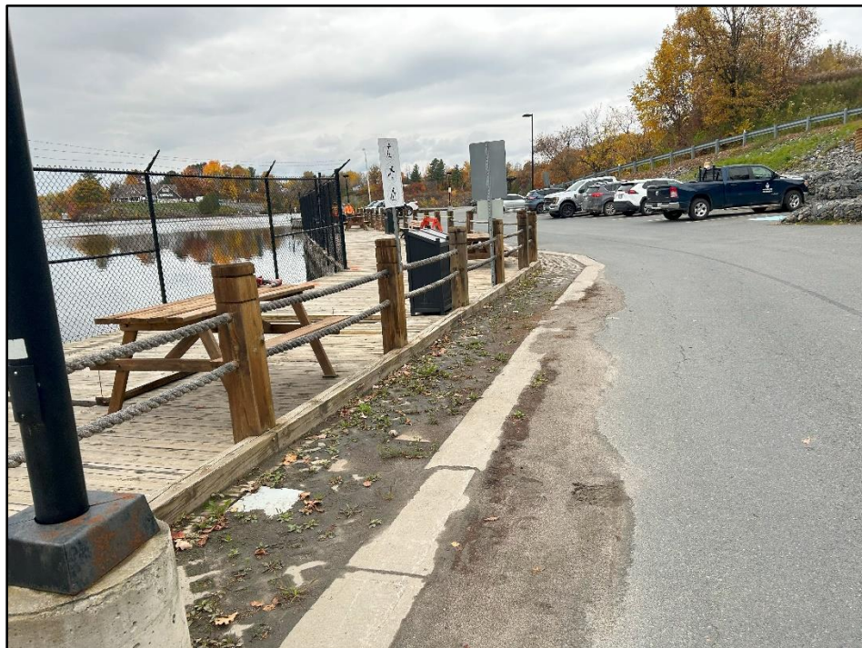
Photo 22: General soil movement at drainage pavers.
